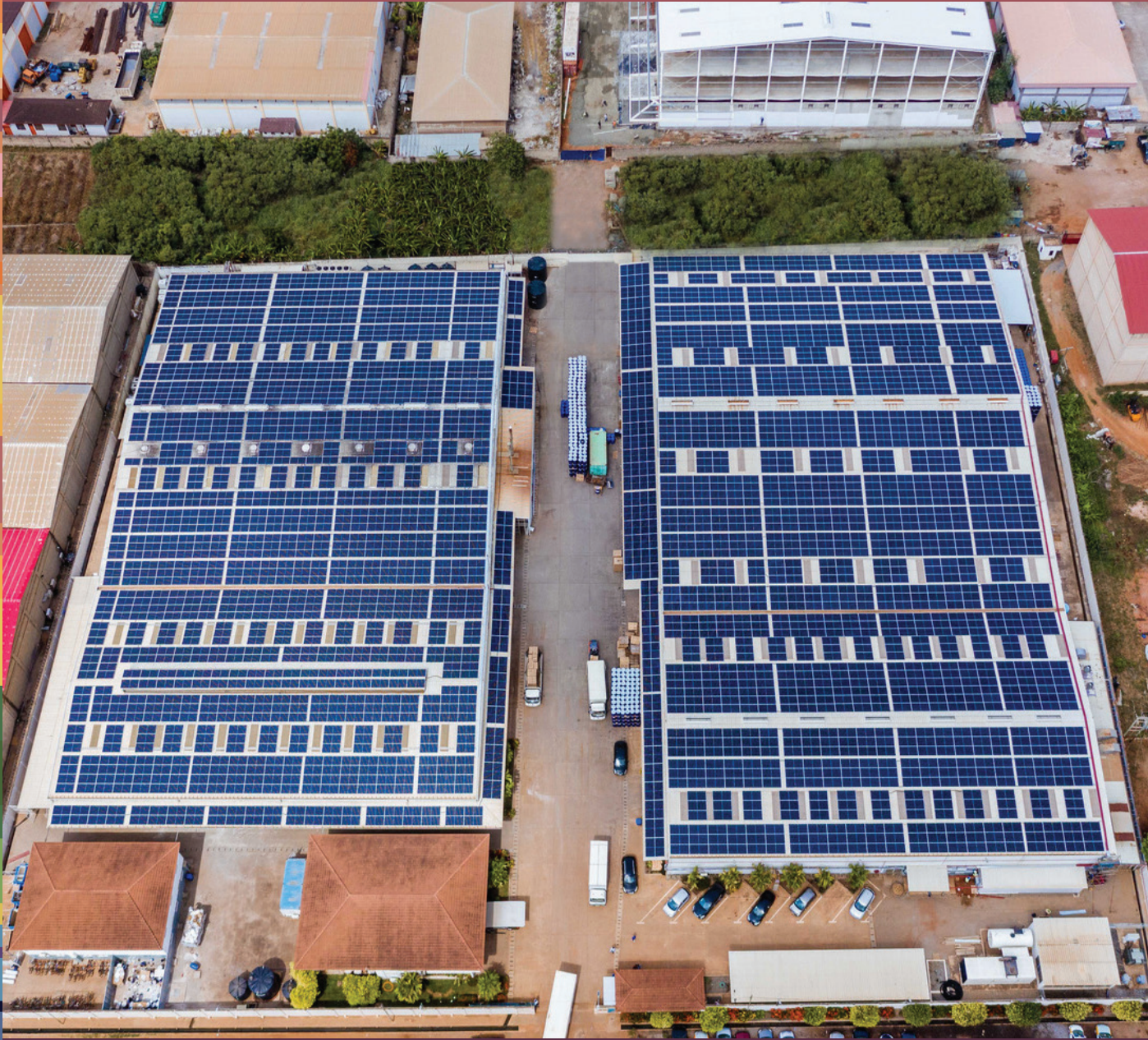
Rooftop solar generation at Chandour Cosmetics Ltd in Accra, Ghana. Photo: © Ghandour
